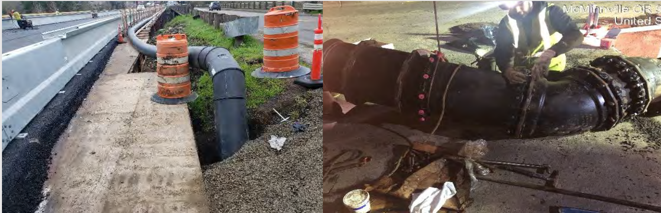
Many Fused Joints and Complex Coupling.
