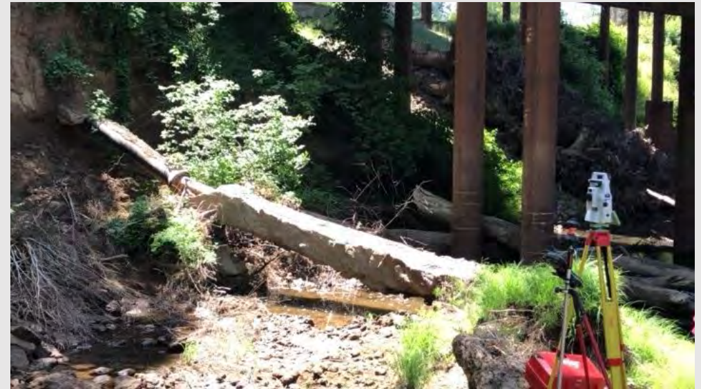
Bank scour exposed the abandoned force main.
