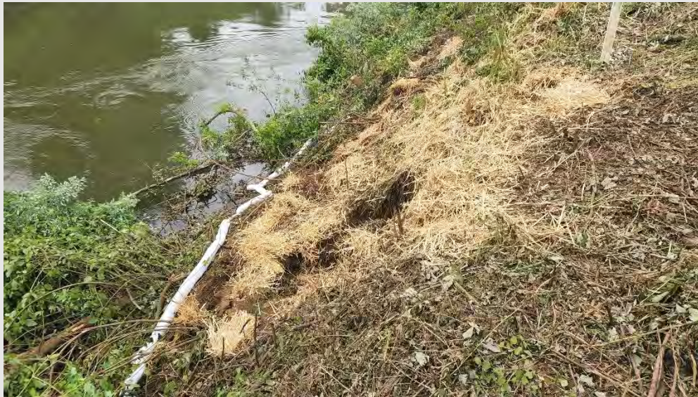
Pile driver found the abandoned force main.
