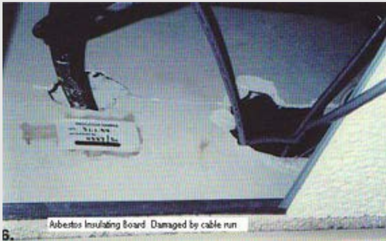
Damage caused by cable
